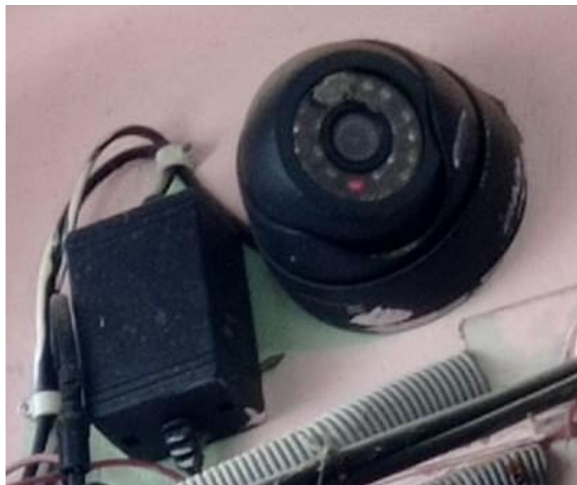
Fig. 6: CCTV surveillance on campus
